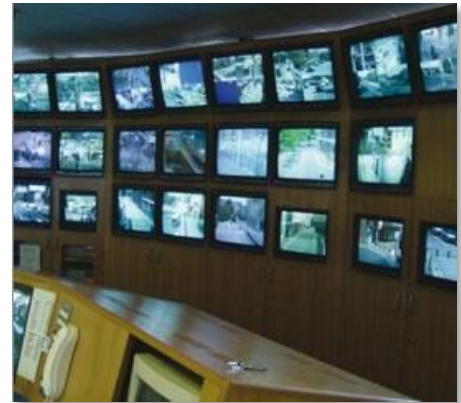
Figure 9 CCTV Operating Room Romford
