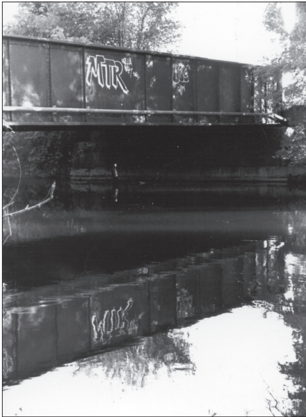
Graffiti offenders risk injury by placing graffiti on places such as this railroad bridge spanning a river.
