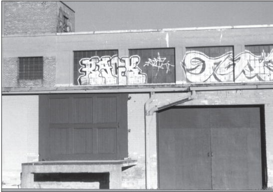
Graffiti often appears in hard-to-reach yet highly visible locations, such as on the upper-story windows of this warehouse.
