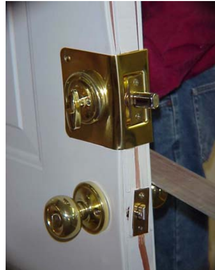
Door edge is vulnerable to splitting
