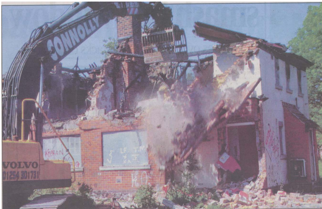
END OF AN ERA: The roof goes first during the demolition of a vandalised and boarded-up house on Crummock Road, Farrington Park
